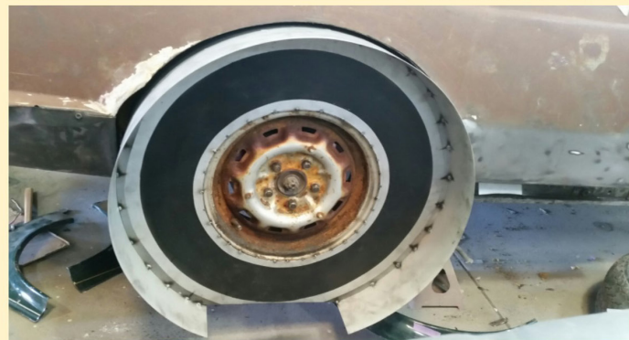
First arch now in place. Modification to the lead edge of under tank panel and rear of sill panel needed to ensure the new profile continues nicely.
